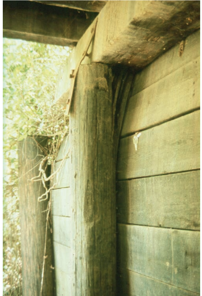
Figure 10.1.36 Local Failure in Timber Pile due to Lateral Movement of Abutment
