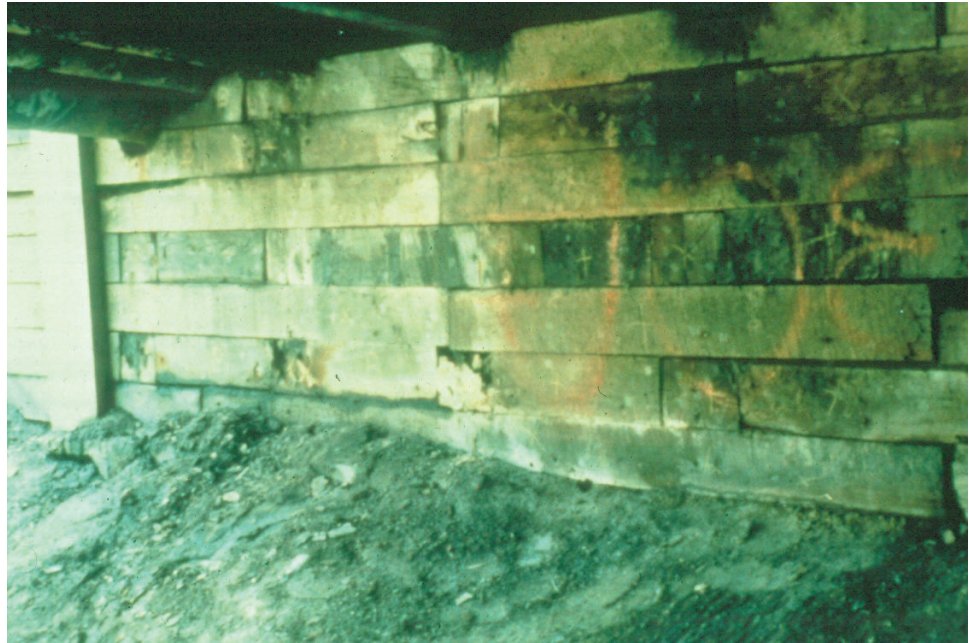
Figure 10.1.37 Decay in Lagging of Timber Crib Abutment
