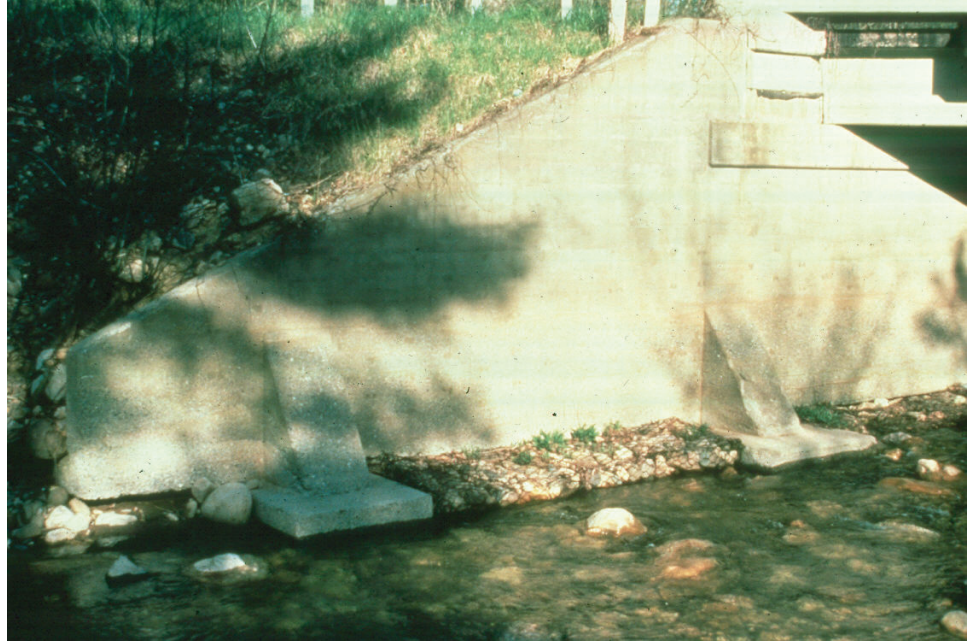
Figure 10.1.51 Scour and Possible Undermining of Concrete Wingwall
