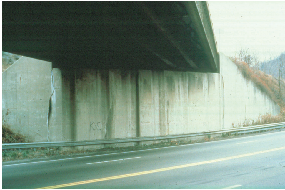
Figure 10.1.53 Settlement Cracks at Integral Concrete Wingwalls
