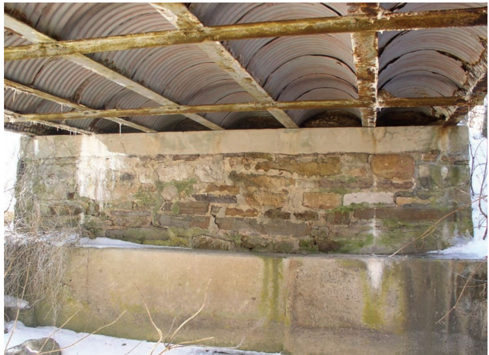
Figure 10.1.32 Cracking in Bearing Seat of Concrete and Stone Abutment
