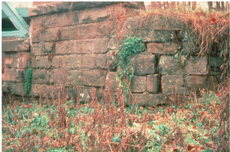
Figure 10.1.54 Deteriorating Stone Masonry Wingwall
