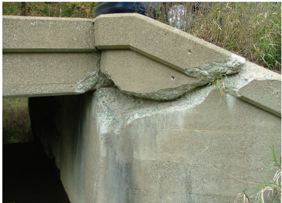
Figure 10.1.50 Deteriorated Concrete Wingwall
