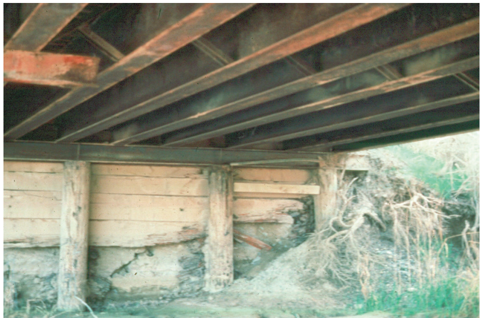
Figure 10.1.38 Decayed Lagging and Scour at a Timber Pile Bent Abutment
