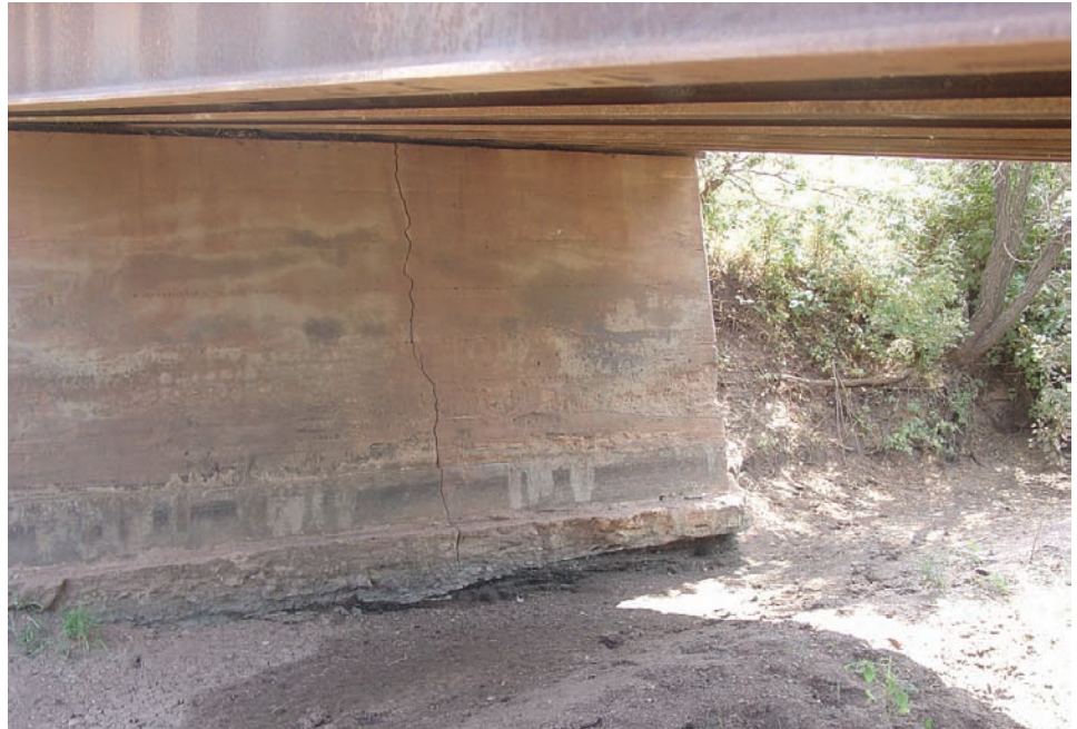
Figure 10.1.24 Crack in Abutment due to Settlement
