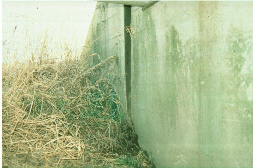
Figure 10.1.49 Rotational Movement at Concrete Wingwall
