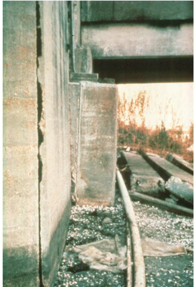
Figure 10.1.30 Rotational Movement at Abutment
