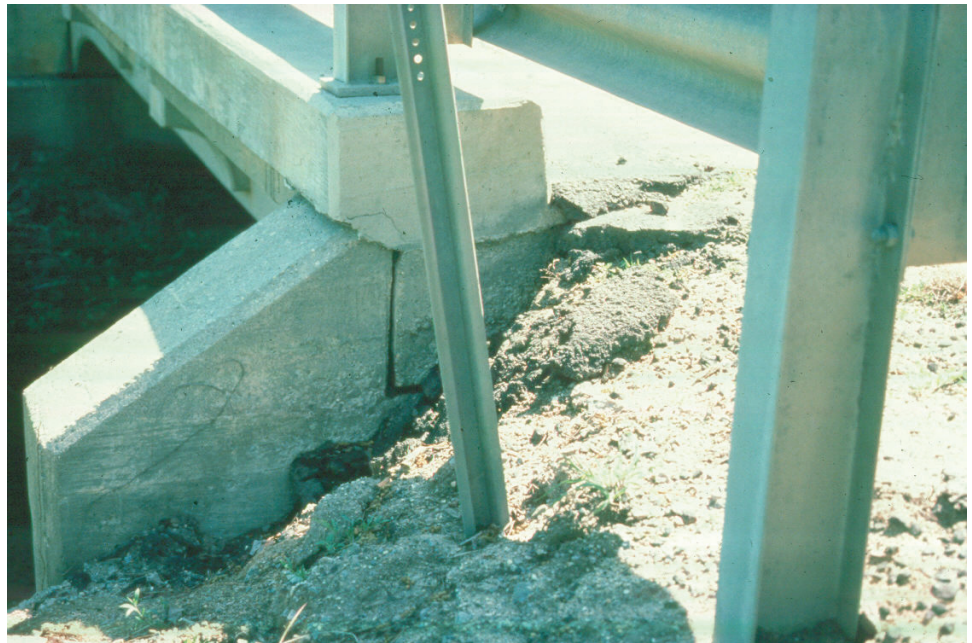
Figure 10.1.52 Roadway Shoulder Erosion Behind Wingwall
