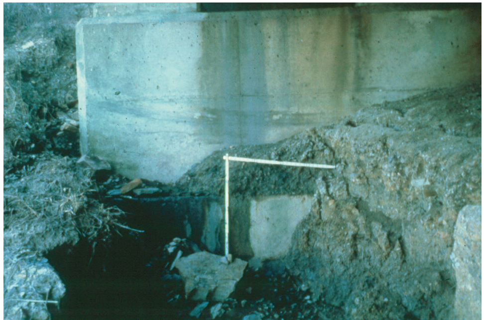
Figure 10.1.28 Erosion at Abutment Exposing Footing
