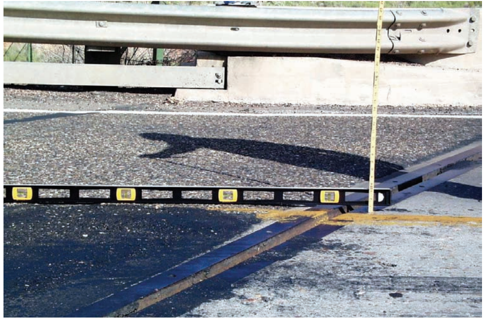
Figure 10.1.27 Depressed Approach Slab due to Rotating Abutment
