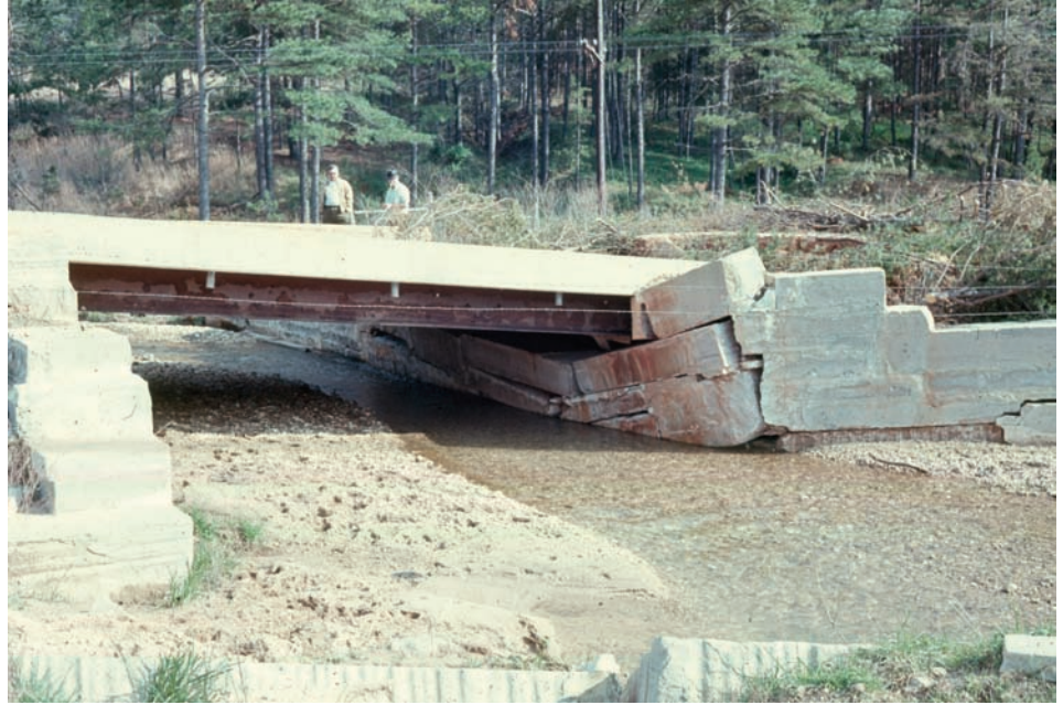
Figure 10.1.39 Abutment with Undermining due to Scour
