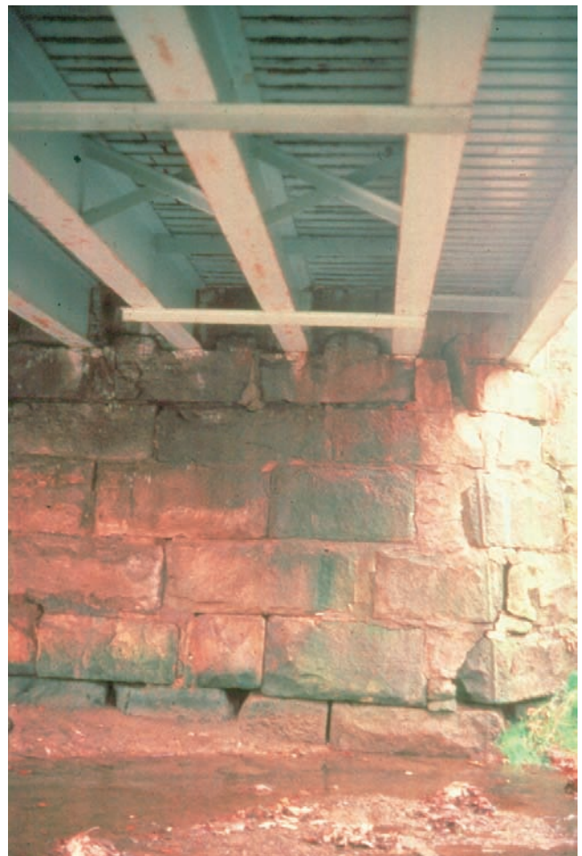
Figure 10.1.34 Deteriorated Stone Masonry Abutment
