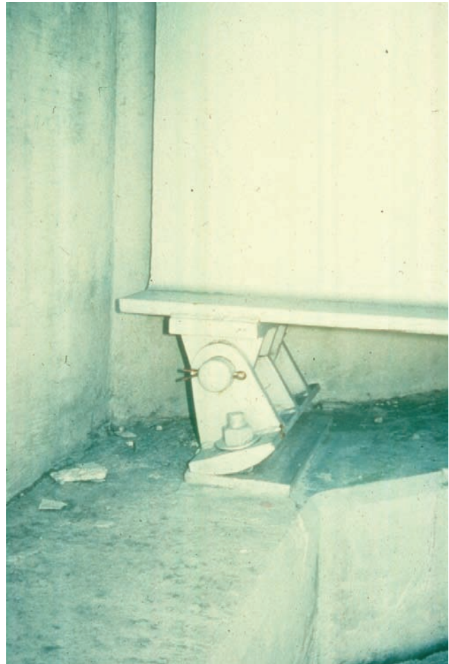
Figure 10.1.26 Excessive Rocker Bearing Displacement Indicating Possible Lateral Displacement of Abutment
